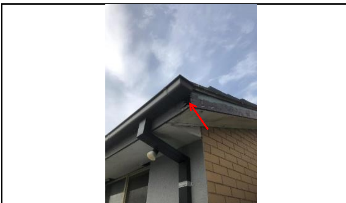
Photograph 4. Example of rot to external timber.
