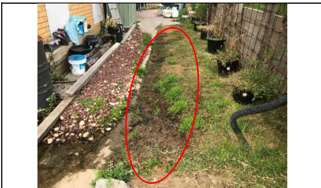
Photograph 3. Wet area observed along the southern elevation of the dwelling.
