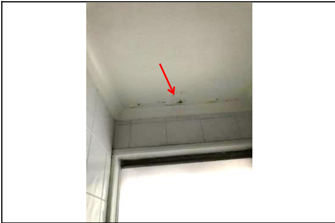
Photograph 9. Example of flaking paintwork to laundry/WC ceiling.
