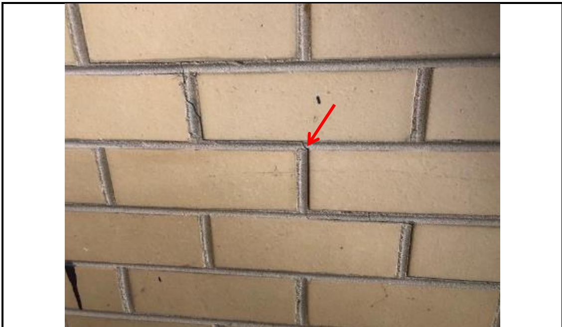
Photograph 6. Example of very slight cracking to eastern elevation brickwork.
