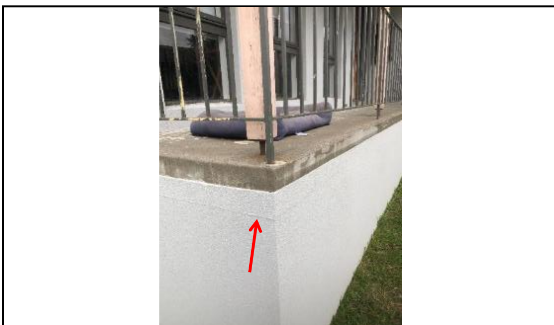
Photograph 12. Very slight crack to north-west corner of dwelling.
