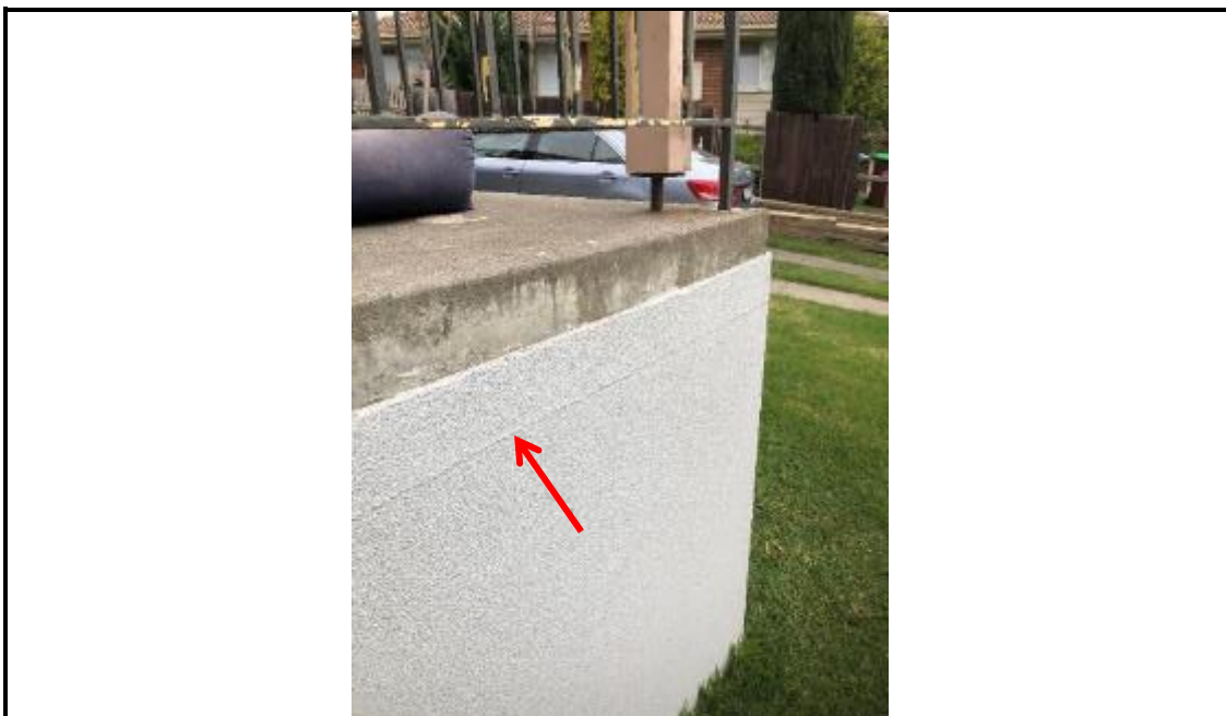
Photograph 10. Very slight crack to north-west corner of dwelling.
