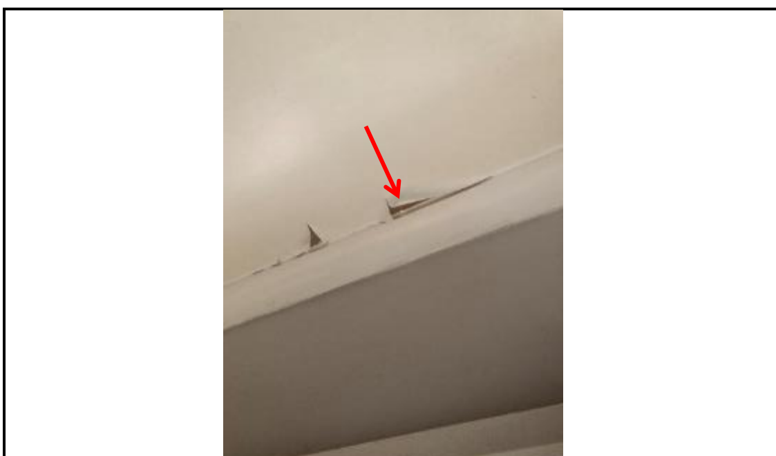
Photograph 8. Example of flaking paintwork to laundry/WC ceiling.
