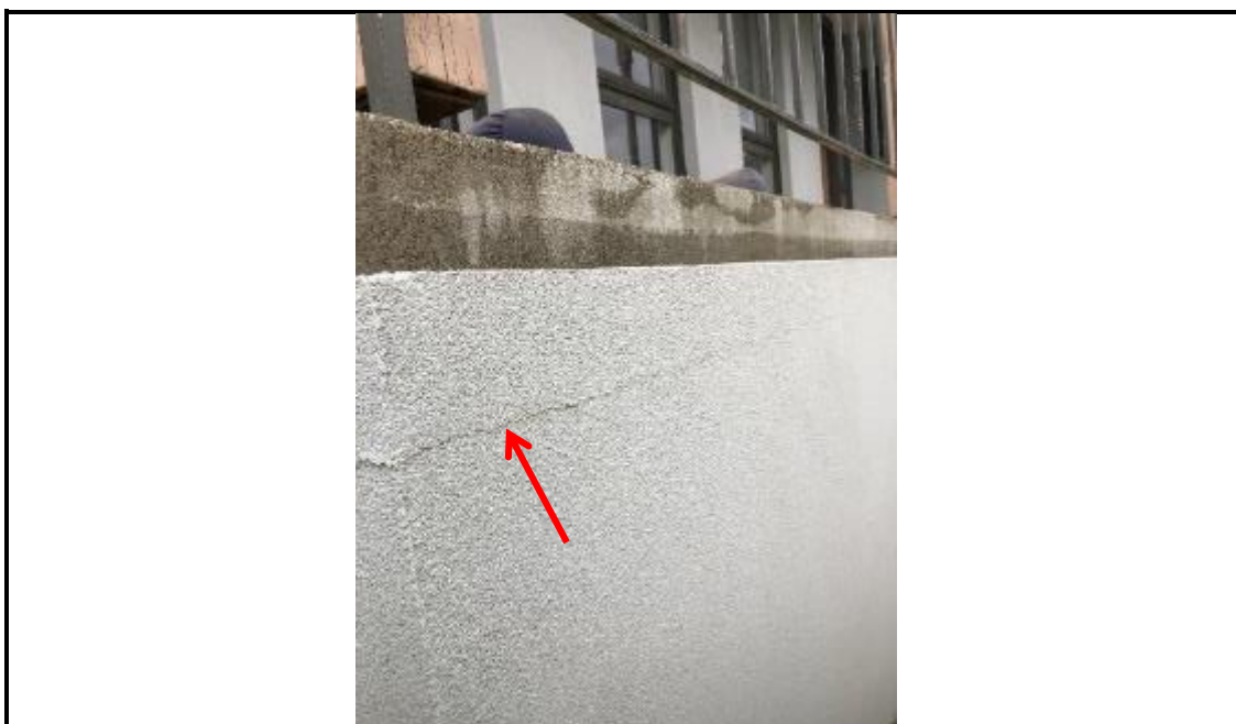
Photograph 11. Very slight crack to north-west corner of dwelling.
