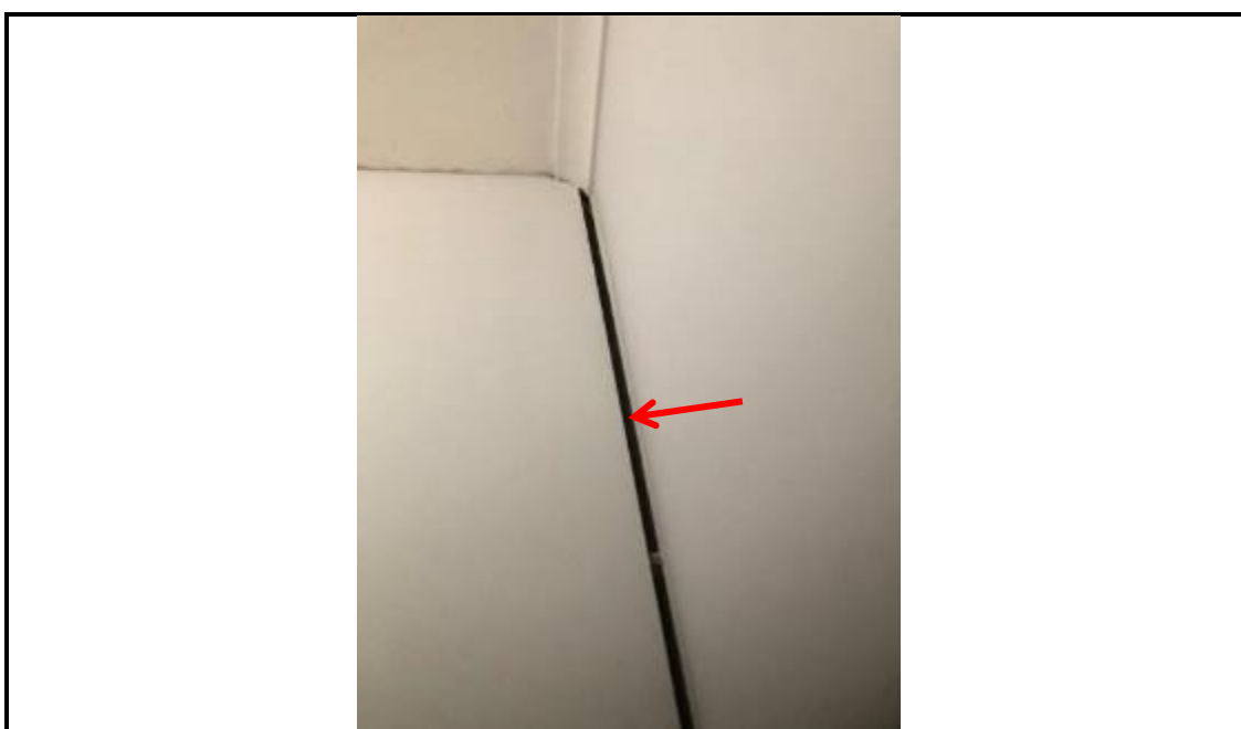
Photograph 14. Gap observed between master bedroom built in robe and adjacent wall.
