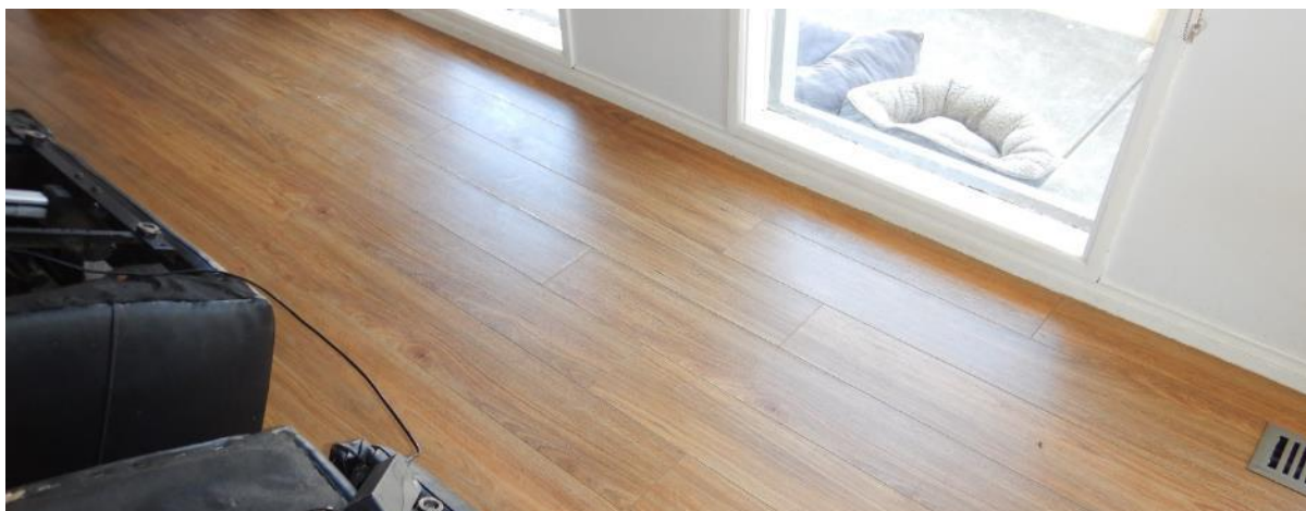
Photo 34 shows the area of the claimed damaged floorboards.
