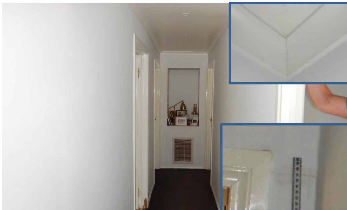
Photo 42 shows a typical view of the hallway, and the inserts show the noted damage.
