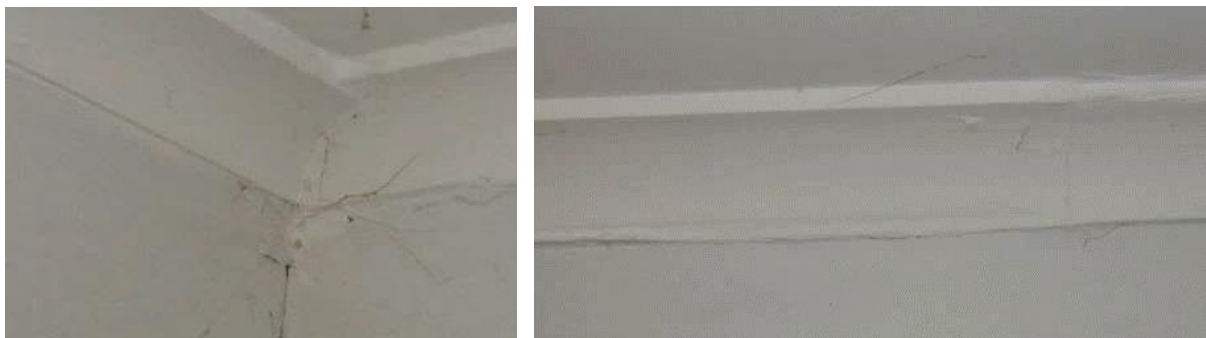
Photos 27 & 28 show a crack along the wall-wall junction and anomalies along the cornice.
