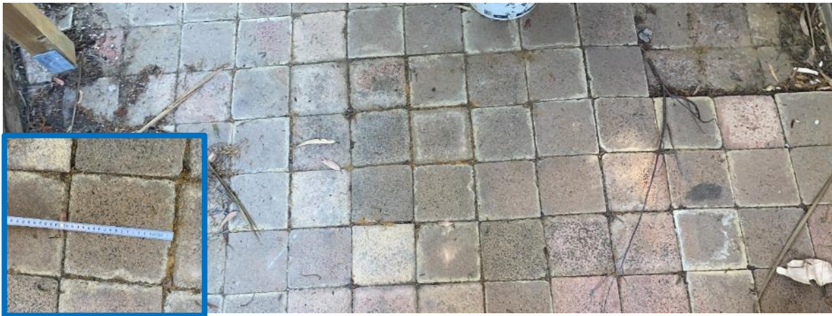
Photo 13 shows undulating pavers along the eastern side of the building.
