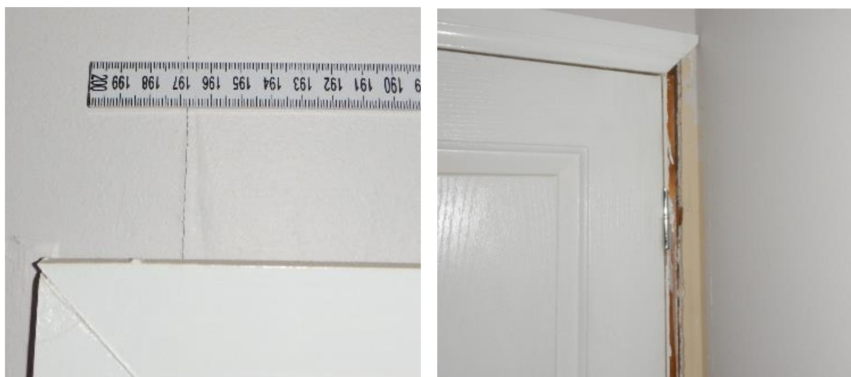
Photos 23 and 24 show the hairline crack in the wall lining and the dislodged casing.
