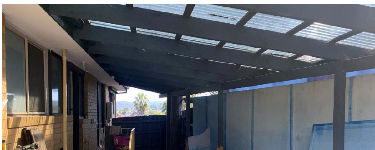
Photo 16 shows a typical view of the underside of the timber pergola structure.
