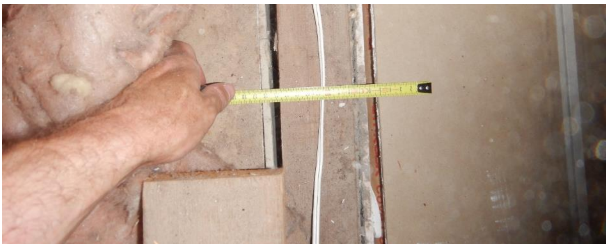
Photo 50 shows the newly installed plasterboard ceiling sheeting (right) and the original plasterboard ceiling sheeting (left) separated by the top plate of a wall frame.
