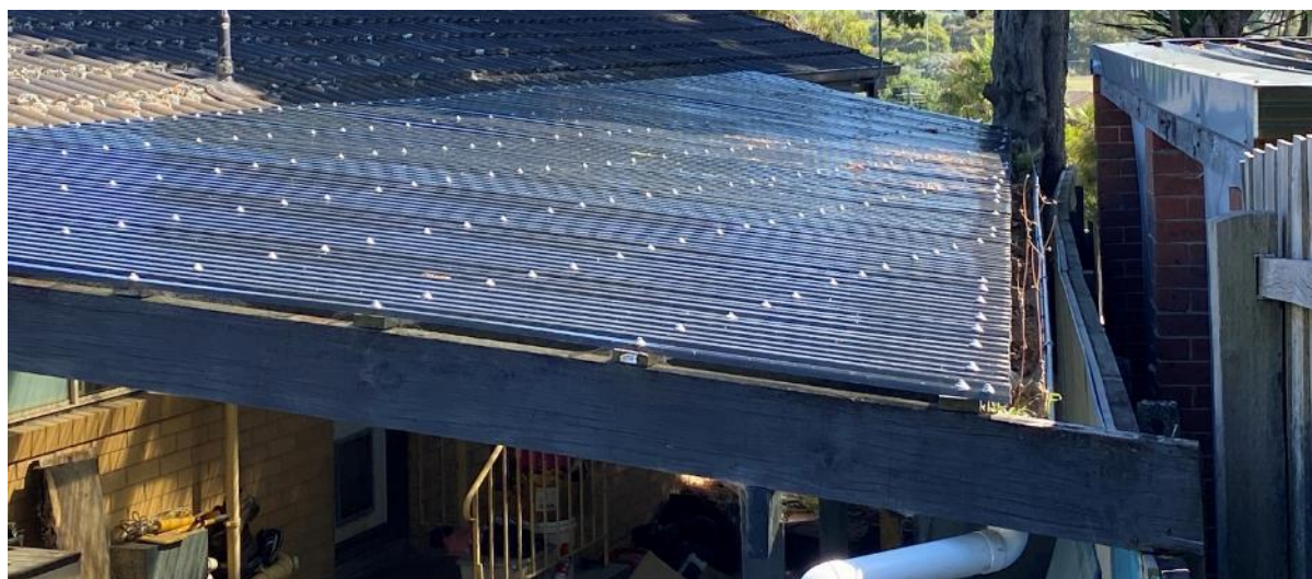
Photo 15 shows a typical view of the sheet roof cladding of the pergola looking north.
