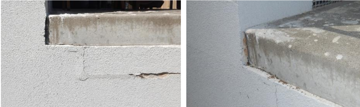
Photos 8 and 9 show the crack and delamination in the porch render and horizontal displacement.
