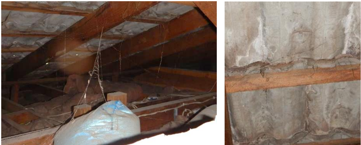
Photos 47 & 48 show daylight through the roof tiles and efflorescence on the underside.
