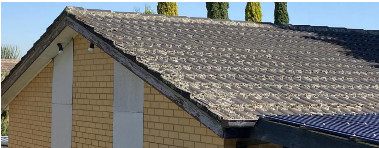
Photo 14 shows the condition of the tiled roof cladding at the south-eastern corner.
