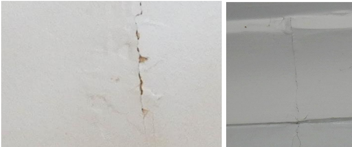
Photos 32 and 33 show a typical view of poor crack repairs and unrepaired cracks.
