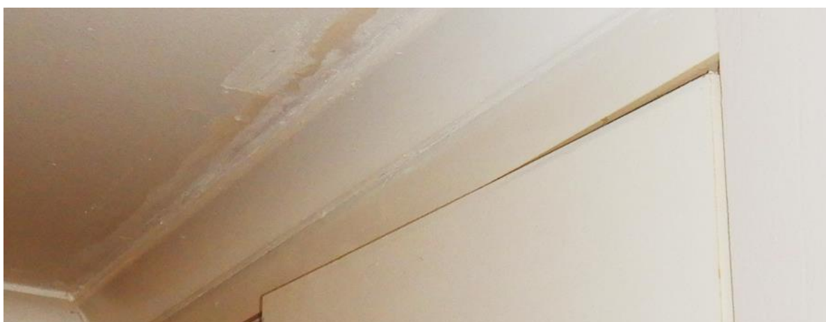
Photo 25 shows poor repair quality in bedroom 3.
