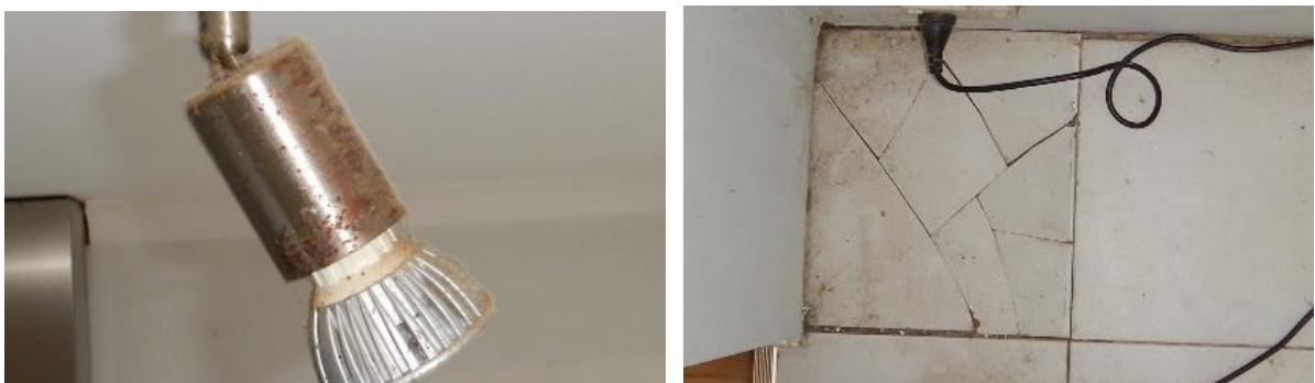
Photos 29 & 30 show rust to the lighting fixture and the damaged floor tiles.
